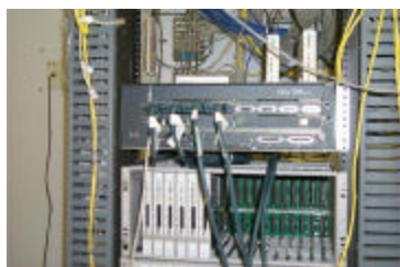
Cisco 7204 Router (PLRCCRTR01)
